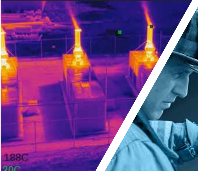
Infrared Thermal Imaging
